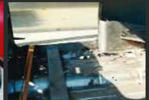
After media blasting it became evident that a new floor needed to be shipped over.
